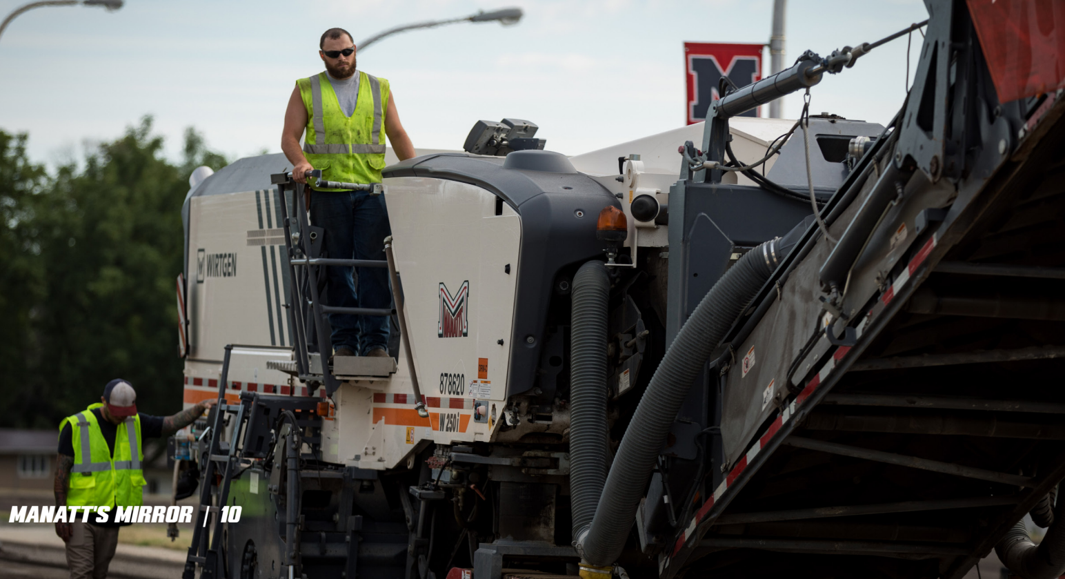
JAMES DAY (BOTTOM LEFT) AND BRANDON HENNING (TOP OF MILL), NEWTON MILLING, MAKING LIGHT WORK OF THE PARKING LOT JOB AT MARSHALTON HIGH SCHOOL
