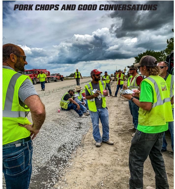
AN UNSEASONABLY COOL DAY FOR THE PAVING CREW IN AUGUST ON HIGHWAY 30 IN STORY COUNTY
